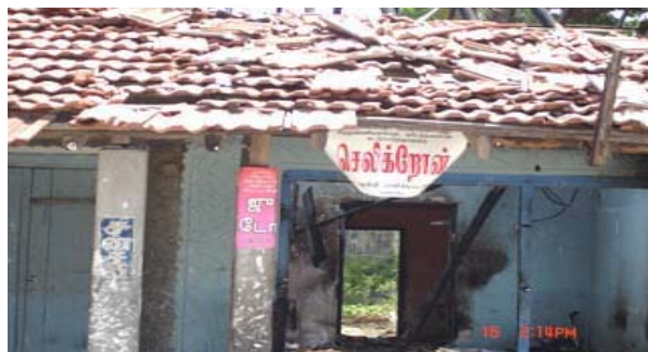
Communication centre damaged by Navy
