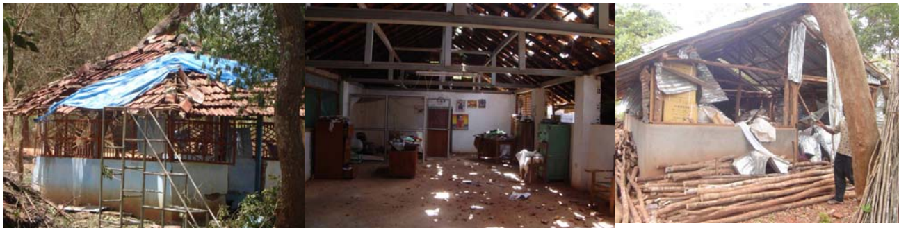
TRO buildings after air strike by SLAF fast attack aircraft in Puthukkudiyiruppu Mullaitivu district.
