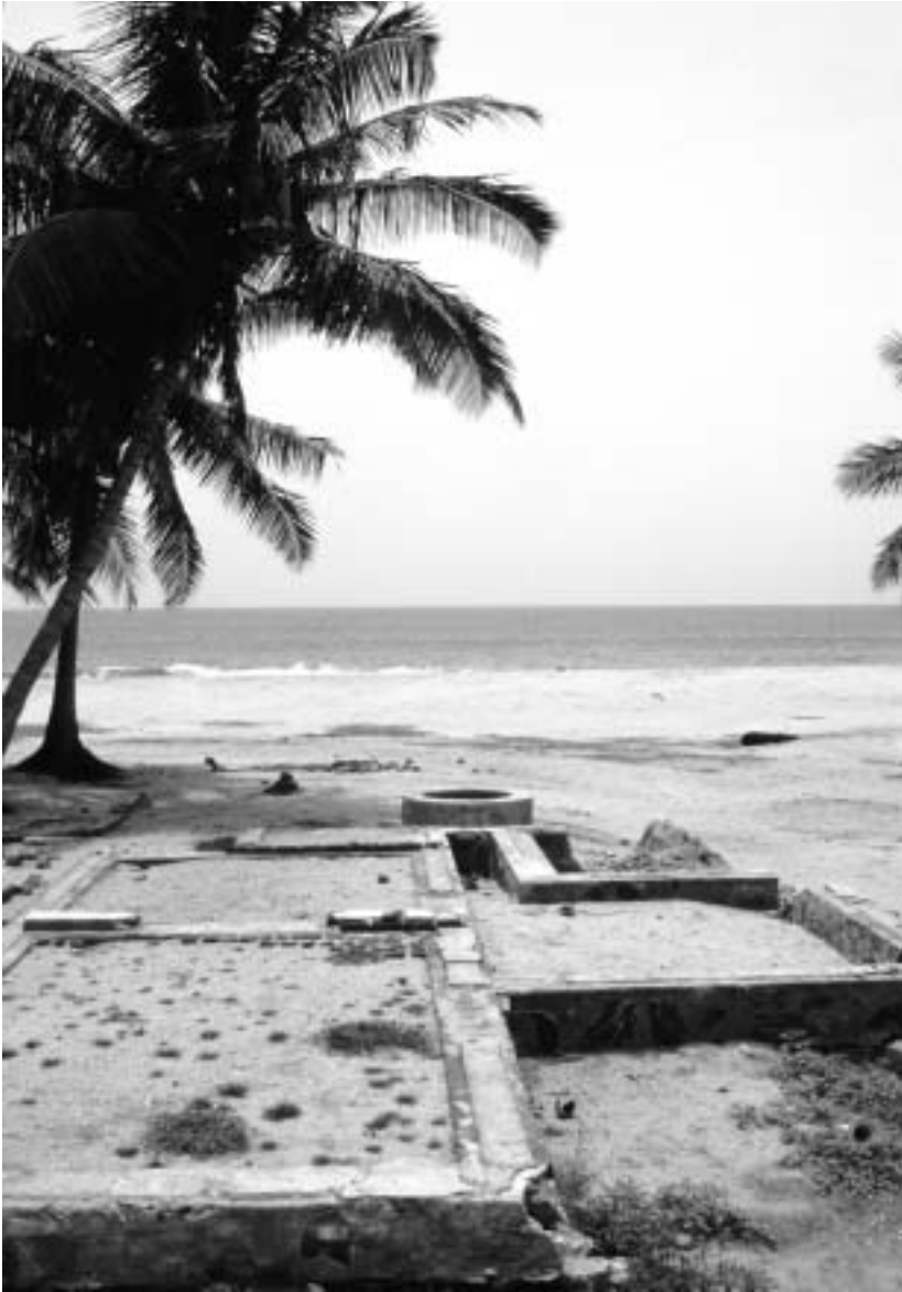
FIGURE 5 BEACHFRONT HOME DESTROYED BY TSUNAMI, MARUTHAMUNAI. AUGUST 2005
